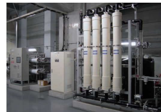
Water-saving cooling water recycling equipment
