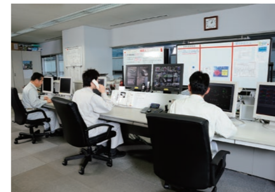
24-hour control room
