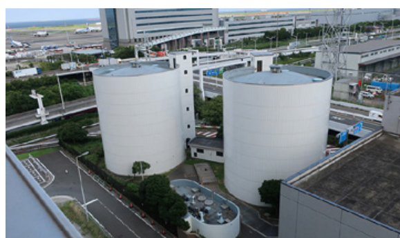
Haneda Airport water supply and drainage facilities
