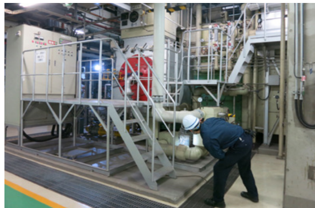
Area heating and cooling system
