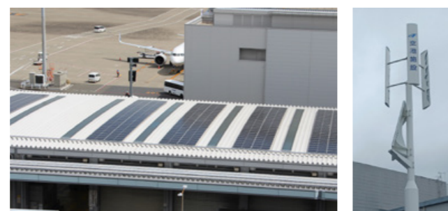
A solar power generation facility for inhouse use in Haneda Airport domestic cargo terminal (left) A hybrid freestanding light (right)
