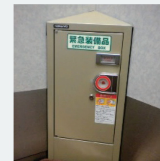
Cabinet in preparation for disaster inside elevators
