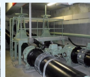
給排水施設 Water Supply and Drainage Facilities
