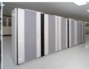
Shared telecommunication server
